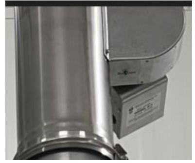
Fig 3.8 Steam Extraction Fan
